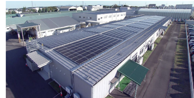
Solar power generation equipment at Product Center in Utsunomiya, Tochigi Prefecture
