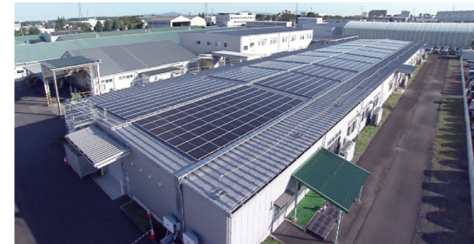
Solar power generation equipment at Product Center in Utsunomiya, Tochigi Prefecture
