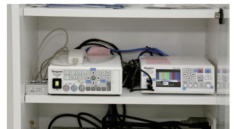
The CCU of MKC-700HD and MDR-600HD installed in the side of a wall
